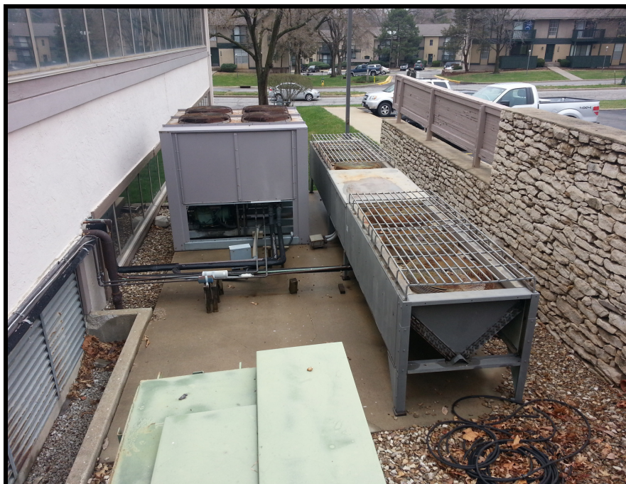
Curry Real Estate Co. – HVAC equipment
